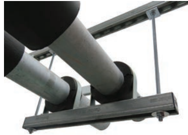
Suspended pipe support
